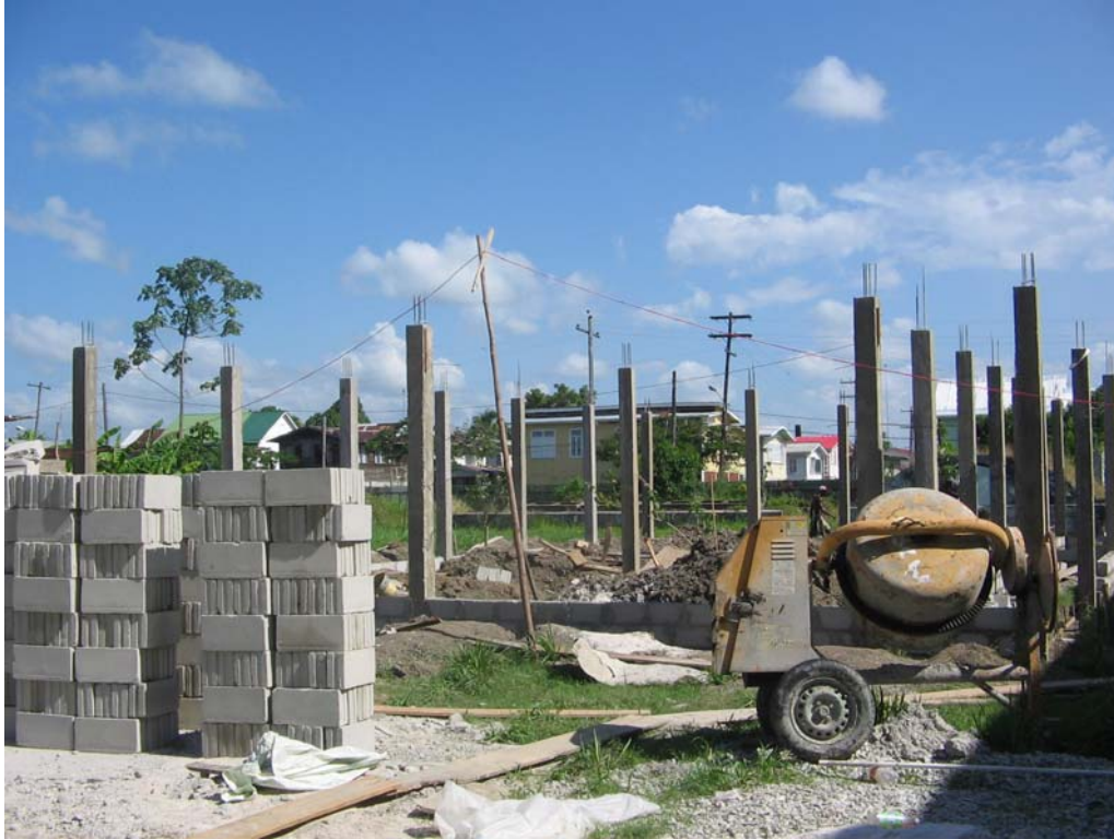
Picture 1: Construction work in progress for new recreational centre Work site photographed on August 12, 2009
