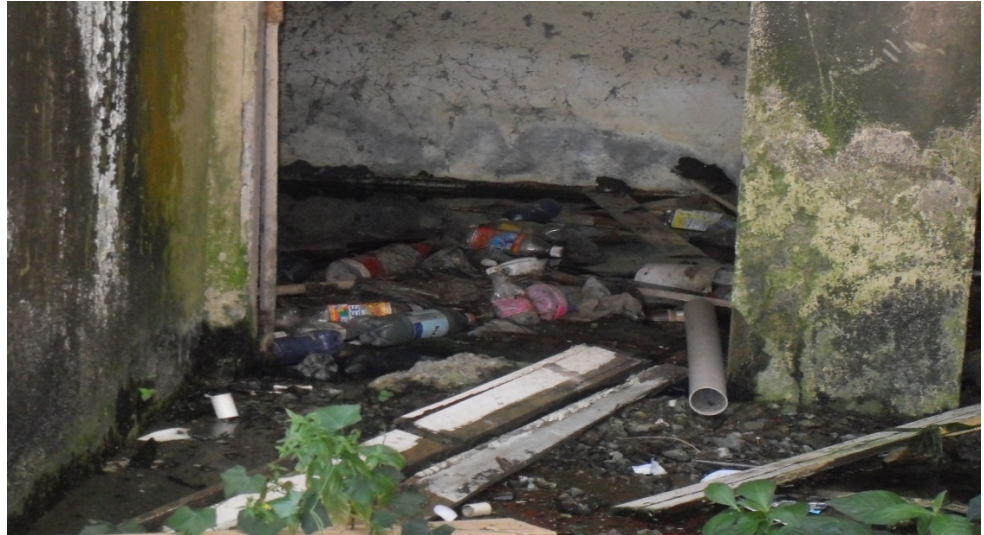
Figure 22 – Unsatisfactory Housekeeping (Photographed 27/ 02/09)
