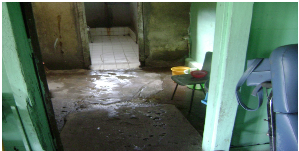
Fig 14 – Water lodged on lavatory floor ( Photographed 14/03/09 )
