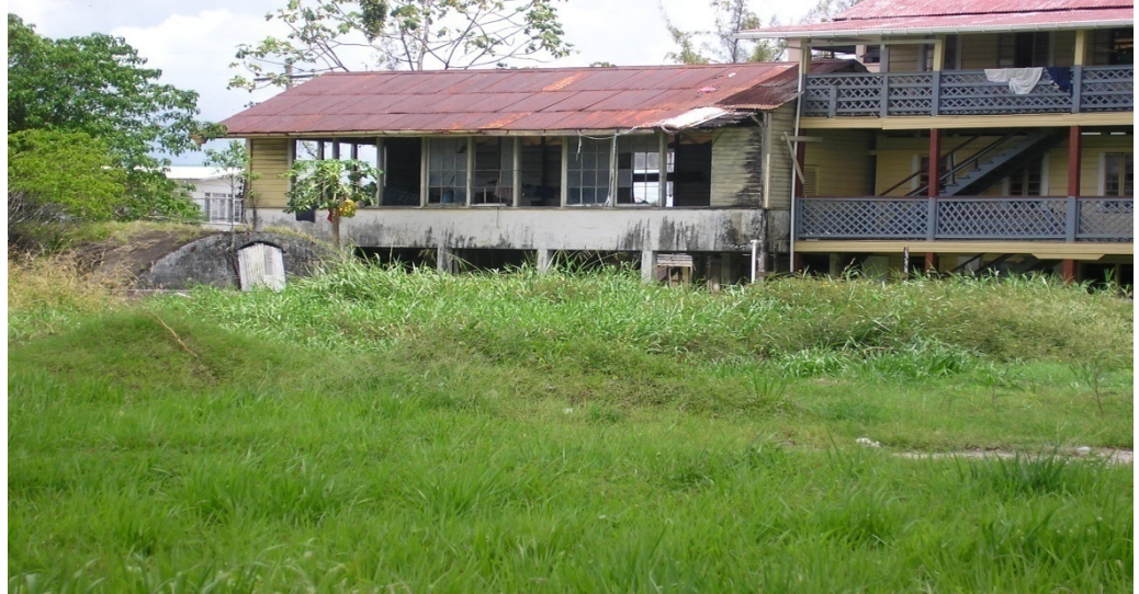
Fig. 17 – Building in need of repairs ( Photographed 14/05/08 )
