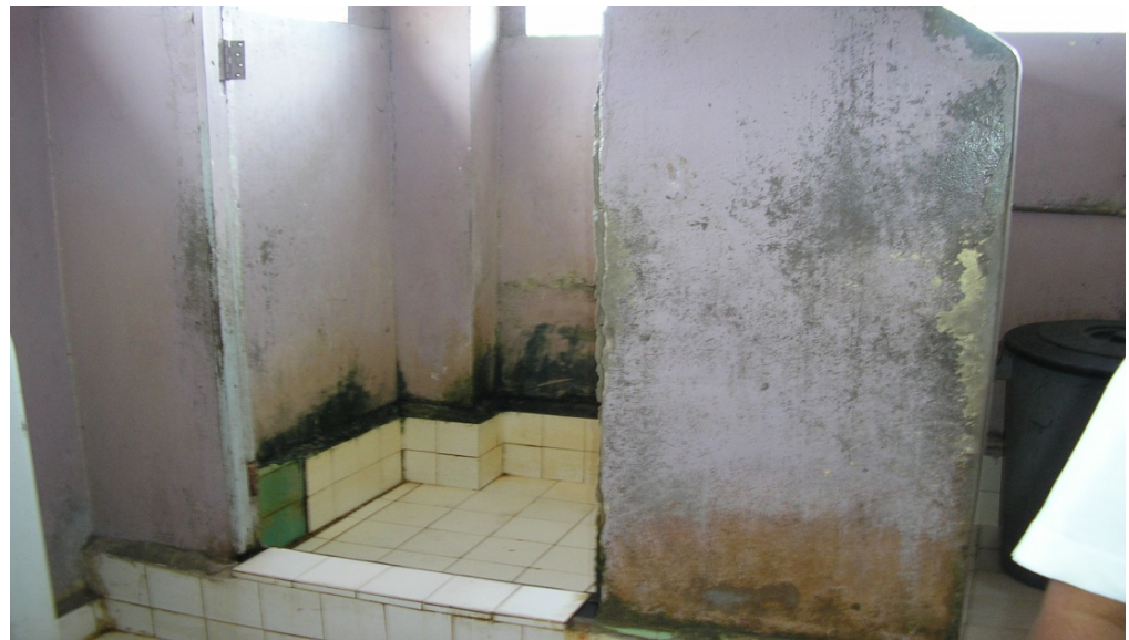
Fig. 19– Dirty and stained bathroom facilities (Photographed 14/05/08)
