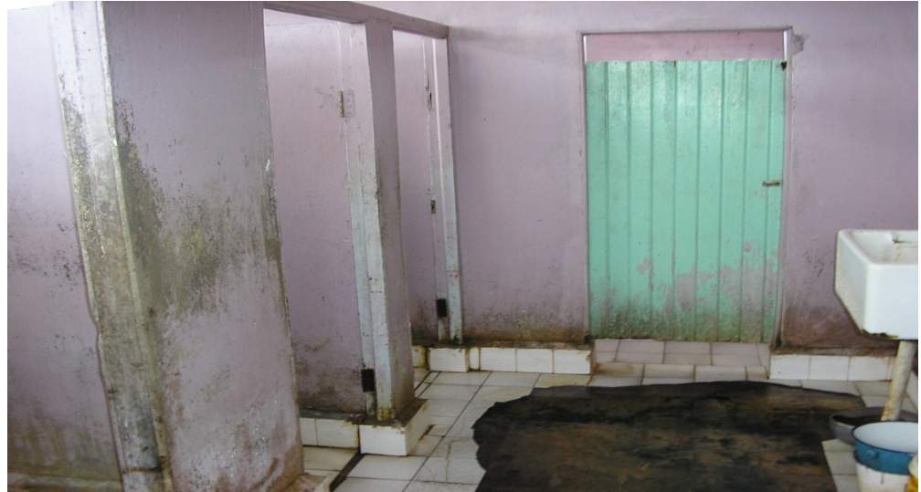
Fig. 18 – Dirty and stained bathroom facilities (Photographed 14/05/08)
