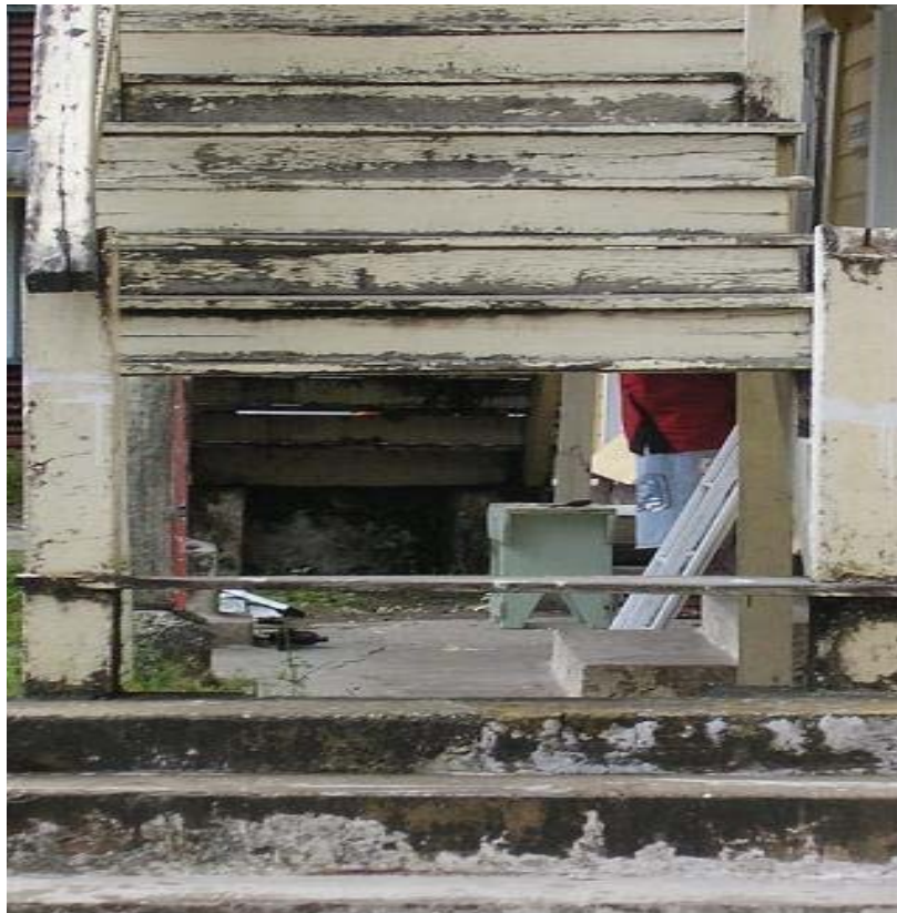
Fig. 21 – Staircase in a state of disrepair (Photographed 14/05/08)
